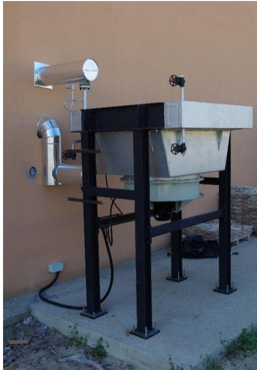
Fig. 5.6 - Air cooler placed outside the laboratory
