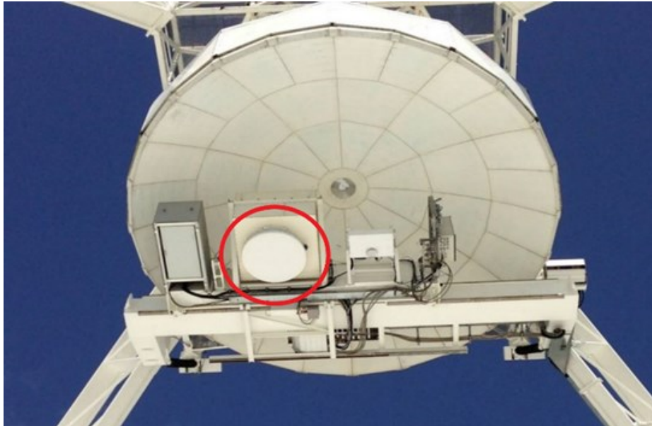
Figure 13 - Picture of the L-P cryogenic receiver (red circled) installed on the SRT primary focus.
