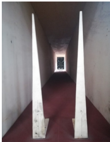
Figure 4. Triangular spires installed at the entrance of the FDS.
