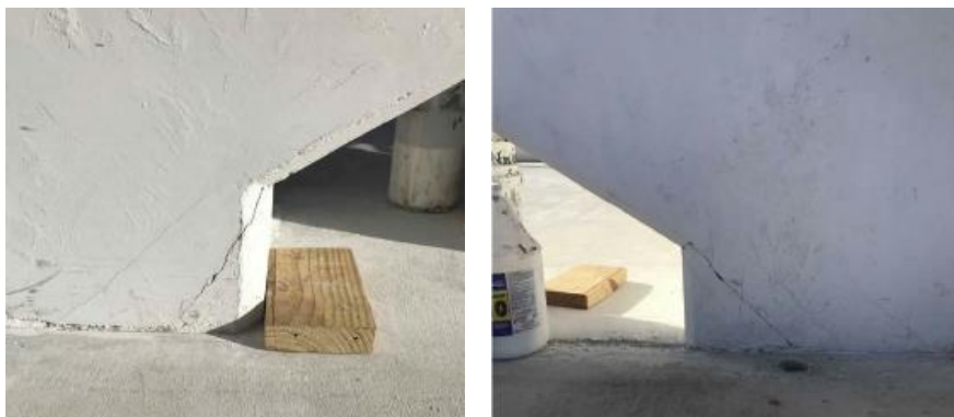
Figure 18: Cracks in node 1, 2 after phase 1 (left) and cracks in node 11, 12 after phase 1 (right).
