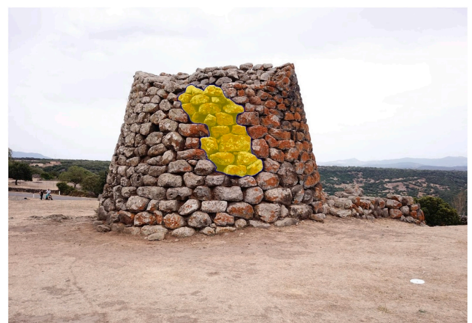
Fig. 2. Nuraghe Sa Jua, criticality area at the stairwell.
