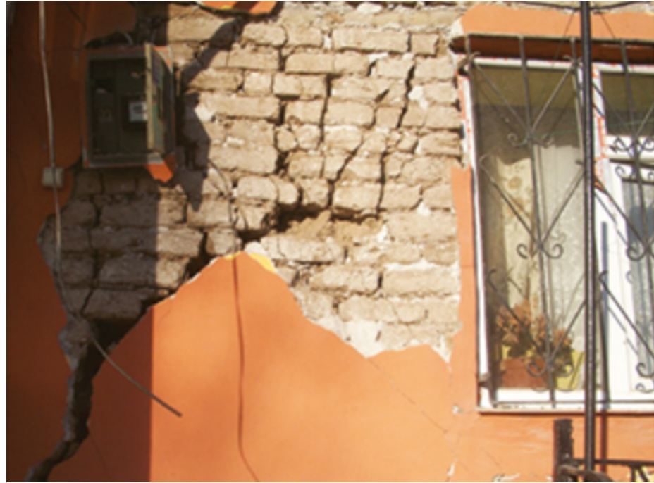
[Figure 4] Example of detachment and sliding failure.
