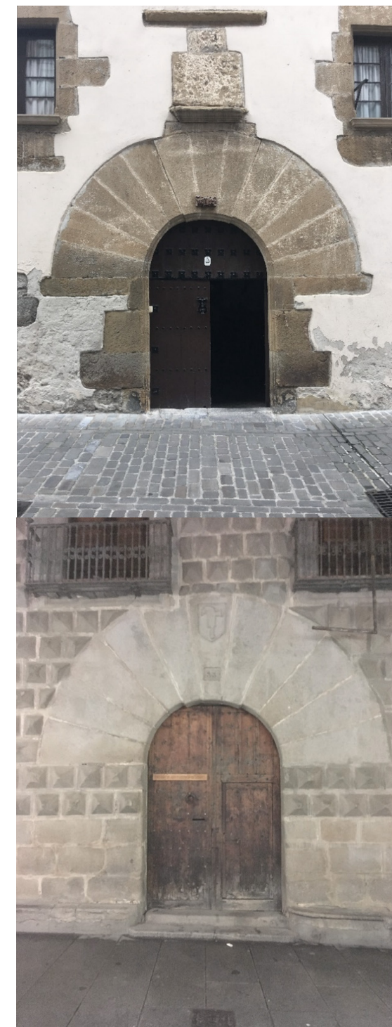
[Figure 35] Examples of thick arches where sliding can be noticed (pictures taken in Segovia, Spain).
