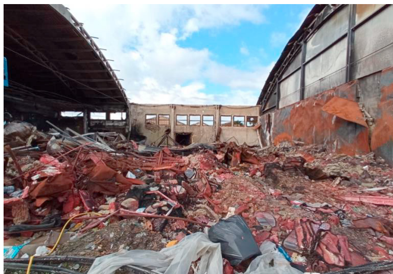
Fig. 1. Warehouse after fire.
