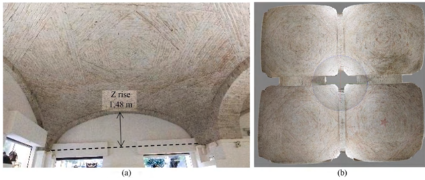
Fig. 1. Typical shallow (lowered) sail vaults in Cagliari: simple (a) and paired (b).
