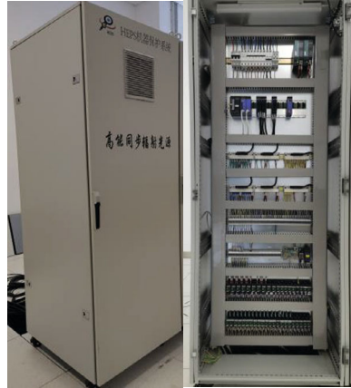
Figure 5.3.8.2: MPS control cabinet of the HEPS.
