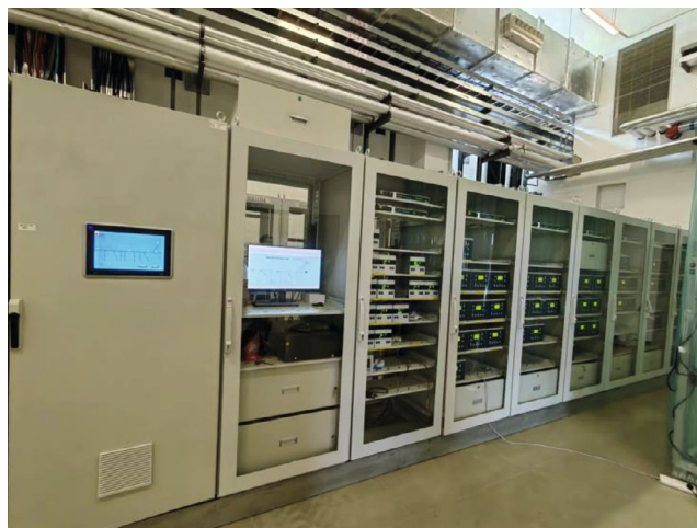
Figure 6.4.8.3: HEPS control and vacuum device cabinets.
