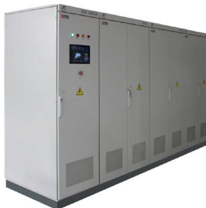
Figure 5.3.4.4: The magnet power supply of the HEPS Booster.
