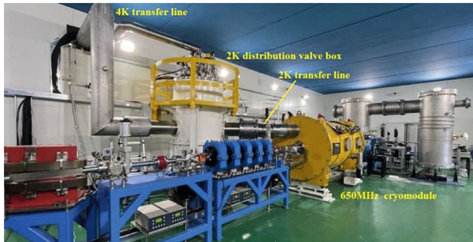
Figure 4.3.1.14: 650 MHz test cryomodule and 2 K valve box.
