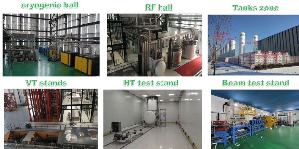
Figure 7.1.23: PAPS cryogenic system for RF cavity R&D.
