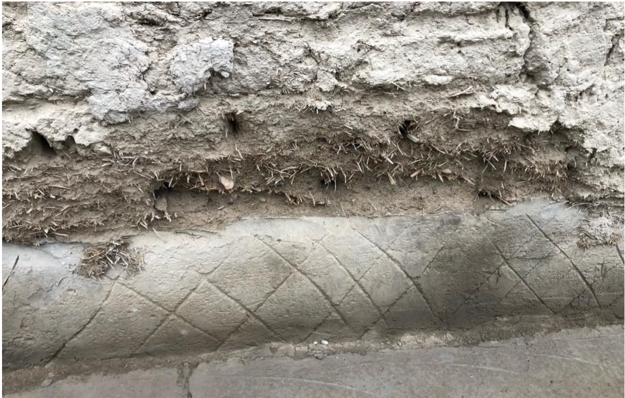
Photo 5. Cement blocks and degradation at the base of the wall. Credits: M. Achenza
