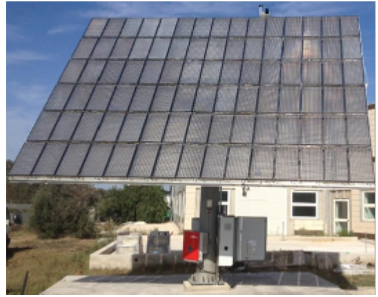
Fig. 1. Case study: HCPV power plant.
