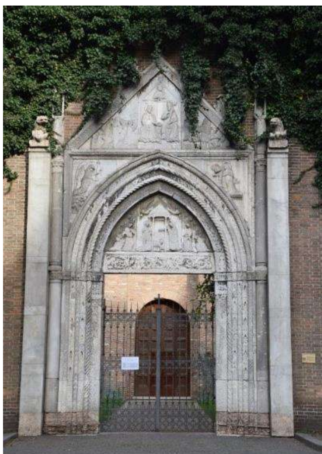
4: Gateway of San Giovanni Evangelista, Ravenna, condition after war damage and reconstruction of 1958 [C. Hoeniger].
