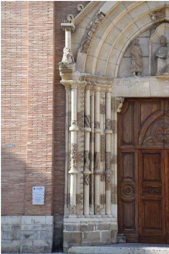
3: Detail of South Portal of San Tommaso, Ortona, attrib. Nicola Marcino di Ortona, 1311-12, after war damage and restoration of 1947 [C. Hoeniger].
