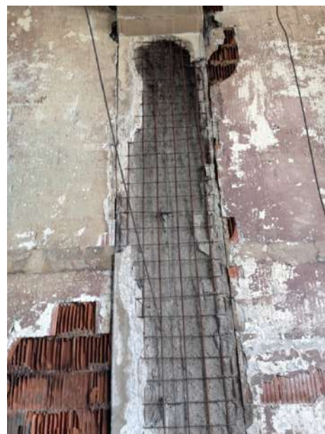
379 380 Figure 13. Column 6 damages.
