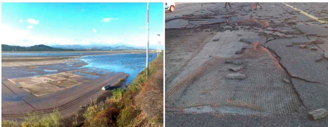
Figure 6. Runway damage after flooding in 2013.
