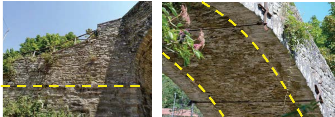
(a) (b) Figure 2: Details of the bridge: wing wall (a) and intrados (b)
