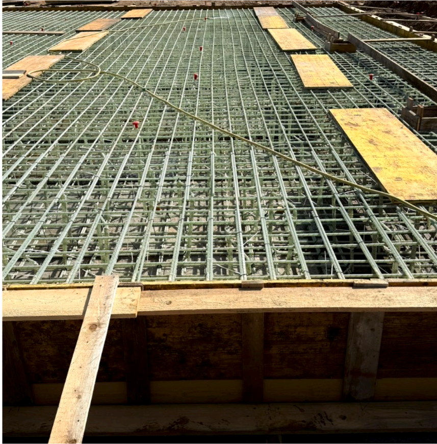
Fig. 5. On-site installation of the GFRP reinforcement cage for the 0.60-m-thick RC raft foundation prior to concrete casting, showing the orthogonal top mesh and detailing over the raft area.
