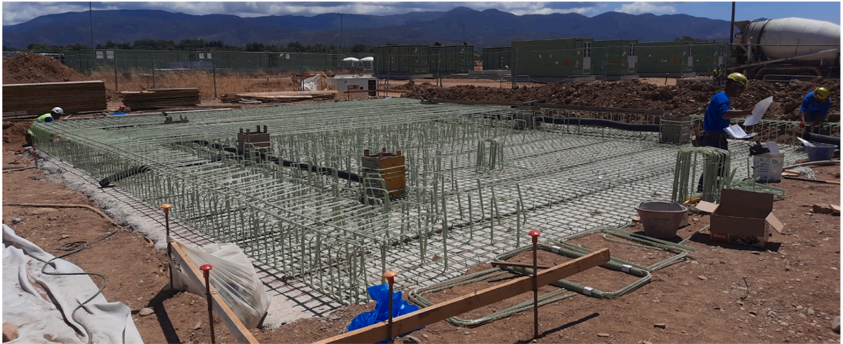
Fig. 7. Construction-stage view of the GFRP-reinforced raft foundation prior to concreting, showing the orthogonal reinforcement meshes and the GFRP chairs/spacers used to maintain the required cover and separation between top and bottom layers.
