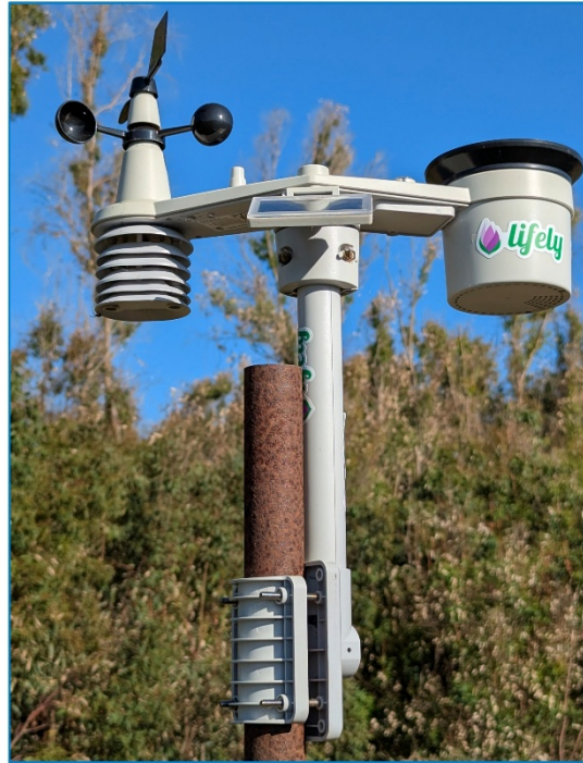
Figure 3.15: SenseCAP S2120 8-in-1 LoRaWAN Weather Station installed on the site.
