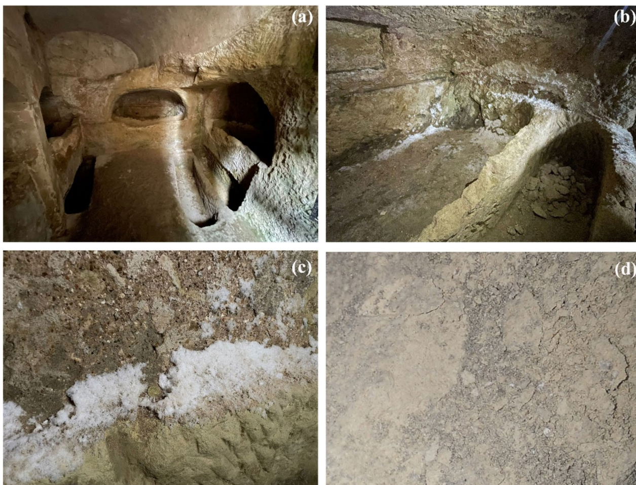
Fig. 1. Munatius Irenaus cubicle (a); material detachment (b); salt efflorescence (c); flaking (d).
