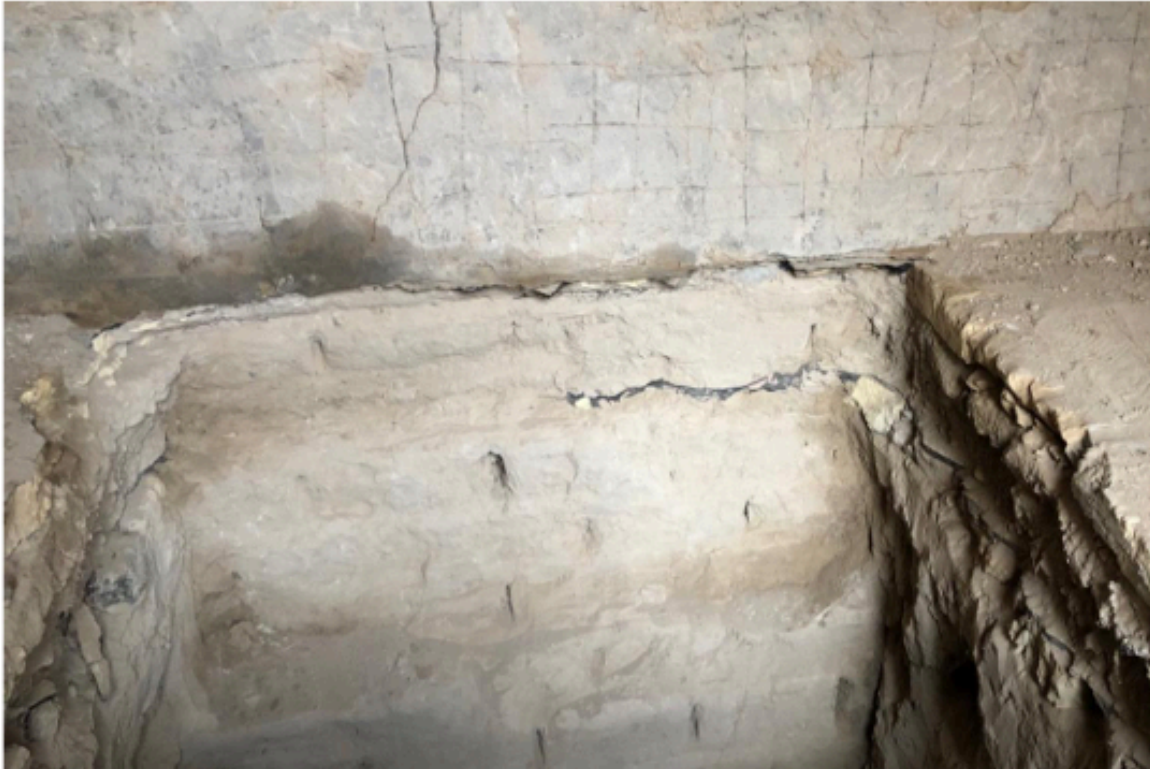
Figure 6. Layers of bitumen in earth masonry at the Ninmakh Temple in Babylon. Credits: M. Achenza
