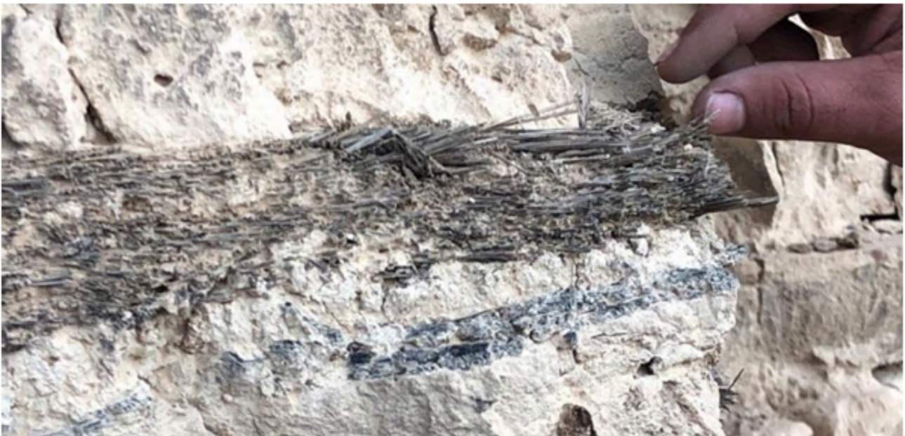
Figure 9. Borsippa: reed mats and bitumen layers in brick masonry. Credits: Ammar Al Taei
