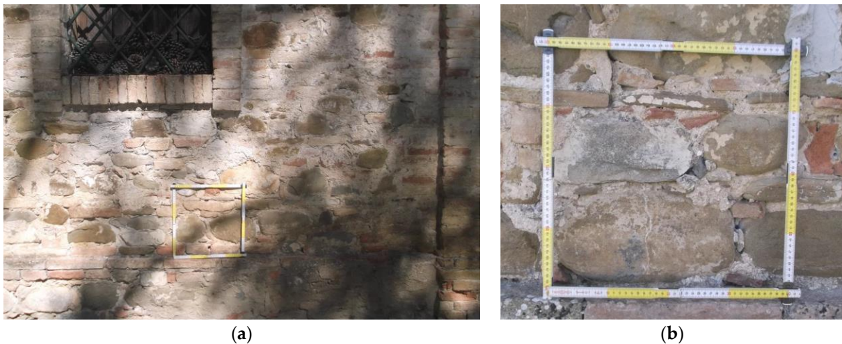
Figure 2. (a) Detail of the masonry walls of the building; (b) Masonry texture (inspection window dimension 40 × 40 cm).
