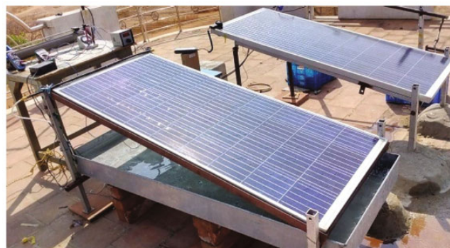
Figure 15. Active cooling: front and back water cooling of a rooftop plant [61].
