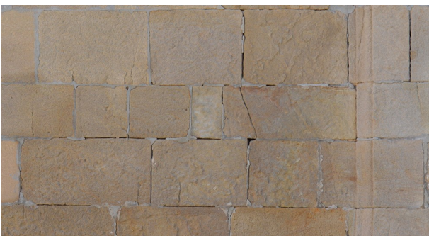
Figure 4. Sandstone masonry of the tower bell, built with the same local material (Pilia E.)
