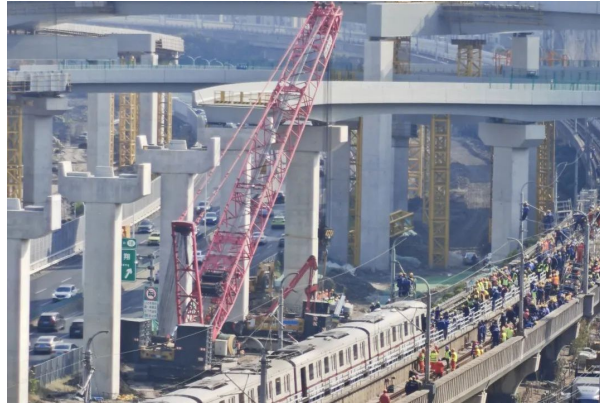
Figure 1.2: Photograph of the 2024 Shanghai Metro Line 11 crawler crane accident site.
