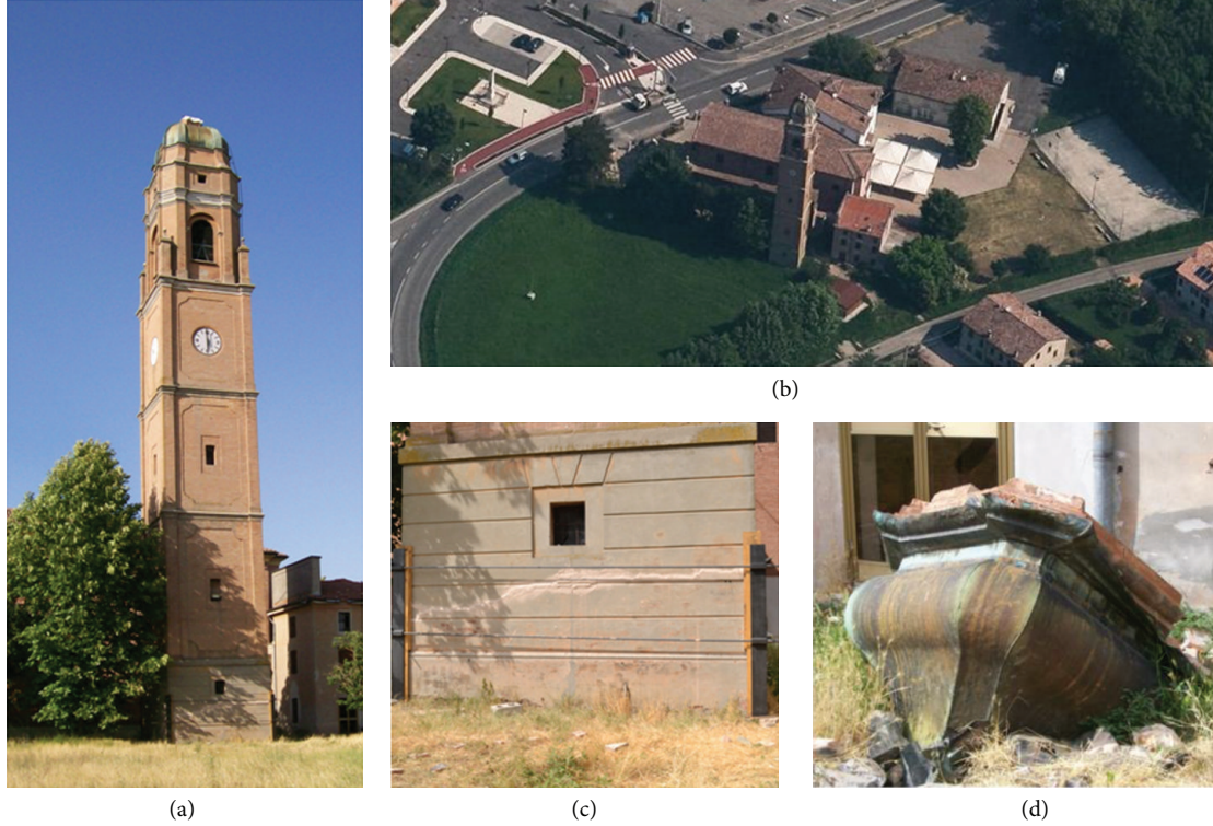
FIGURE 1: Some images of the damaged bell tower. (a) Southwest side of the building. (b) Panoramic view. (c) Cracks at the base of the tower. (d) Collapsed top.
