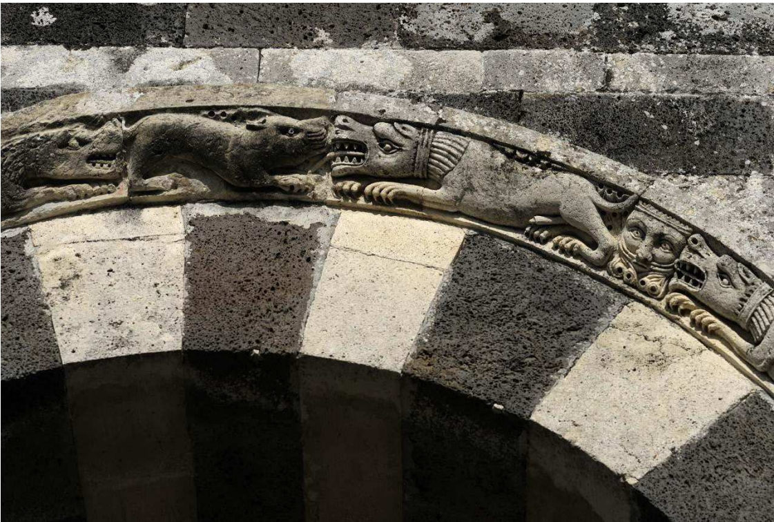
Fig. 3 – Trinità di Saccargia abbey. Detail of the sculpted frieze on an arch in the portico. The right part (both the ashlar and the frieze) has been substituted and recreate during late 19th century restoration works.
