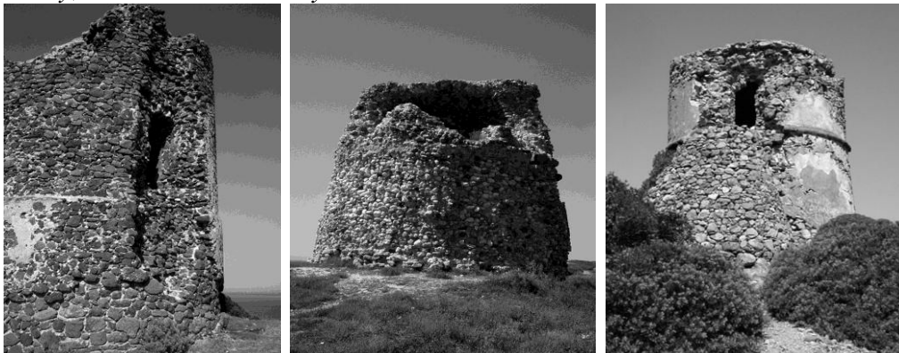
Figure 6. Foghe, Su Puttu and Iskra Ruia Towers. All These Examples Are in Bad Conditions, because Neglected. All the Images Put in Evidence the Various Questions of Degradations, i.e. Erosion, Alveolization, Anthropical Decay, Structural Instability. Photos: S.M Grillo
