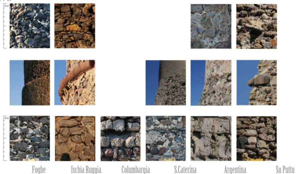
Figure 4. Details of Masonry Referring to Some of the Towers Investigated. The Comparison Highlights the Different Masonry Textures that Characterize the Basis and the Upper Body of Each Tower and the Constructive Solution Adopted for the Connection between the Two Bodies. Graphic Realization: S. Murru
