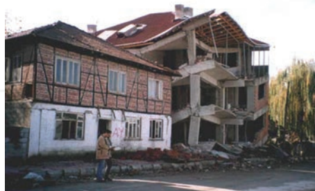
Figure 1. Different damaged conditions of traditional wooden and reinforced concrete buildings after the 1999 Duzce earthquake. Image taken from [6].
