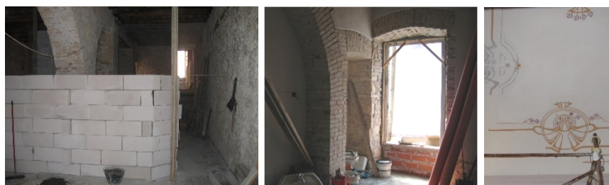
Figure 10: Worksite for the conversion of a traditional house into a bed and breakfast accommodation.
