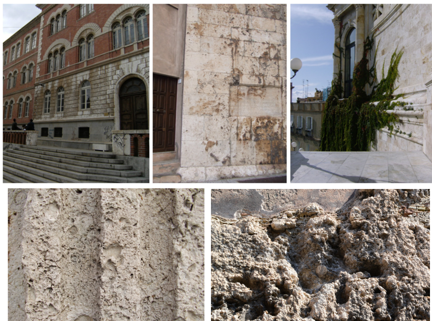
Figure 9: Weathering damage black crusts, biotic alteration, alveolization.
