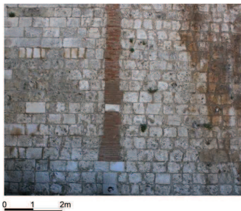
Fig. 7- Rectified photography the shows a part of the west flank of the bastion of Santa Croce . We can observe the original materials adopted in the sixteenth century and characterized by a unique dimension
