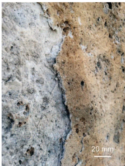
Fig. 8- Compact limestone ashlar of Santa Croce's wall facade, with evident exfoliation and pitting processes and detachment of flake with thickness about of 5 mm
