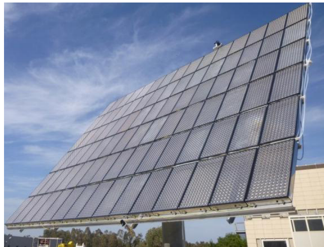
Fig. 3. Solar tracker unit.
