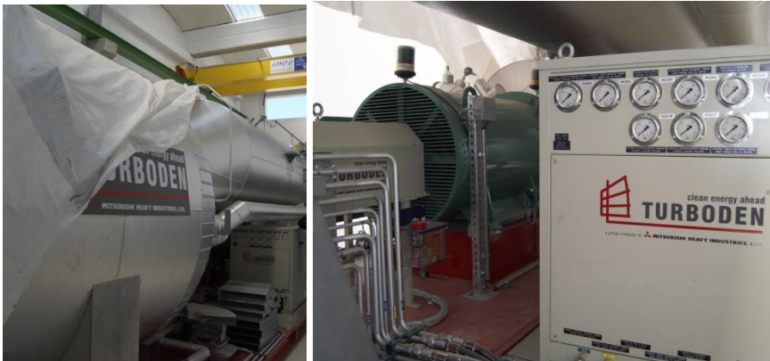
Figure 3.7. ORC power unit of the Ottana Solar Facility.
