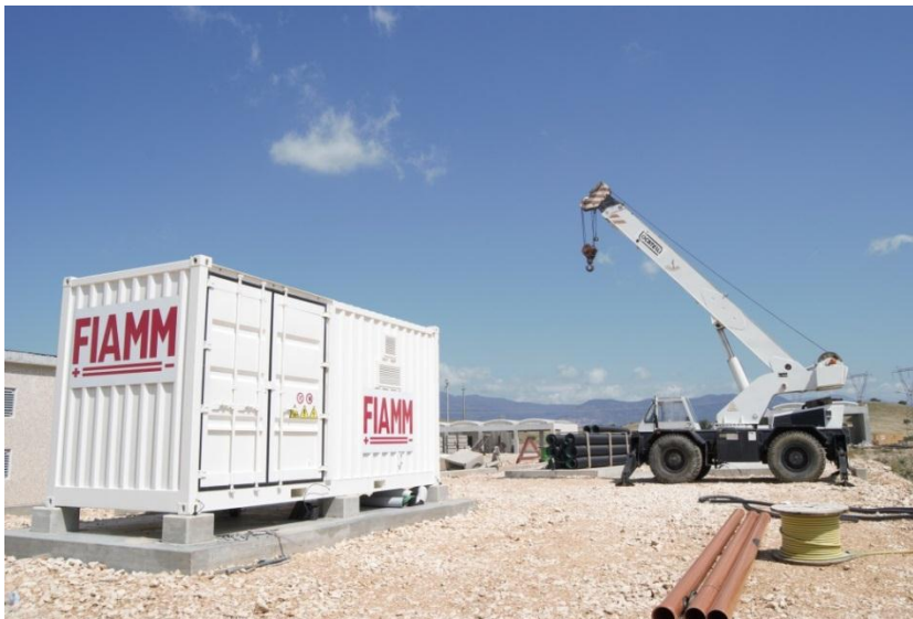
Figure 3.10. Sodium-Nickel battery bank of the Ottana Solar Facility (under construction)
