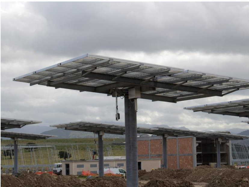
Figure 2.8. High Concentrating Photovoltaic (Ottana Solar Facility)
