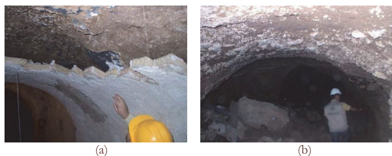
Figure 10: Qualitative survey of the hypogeal structures: assessment of the structural status (a); material and humidity level (b).
