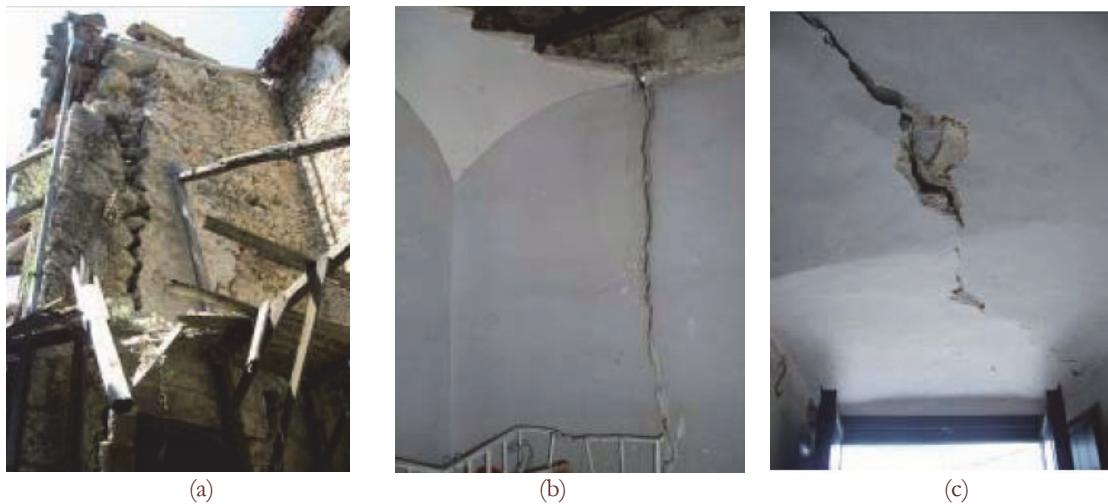
Figure 9: Masonry façade overturning (a); partial vault collapse (b); deep vault crack due to shear action (c).
