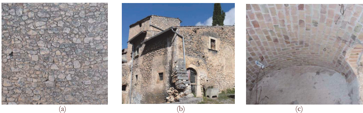
Figure 4: Old masonry texture (a); typical house in the city centre (b); masonry vault (c).
