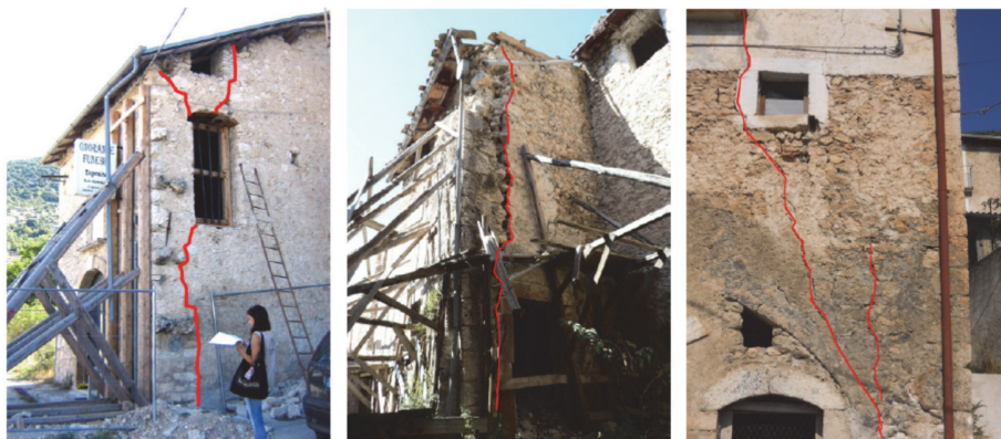
Figure 16: Observed building damage mechanisms, San Pio delle Camere.
