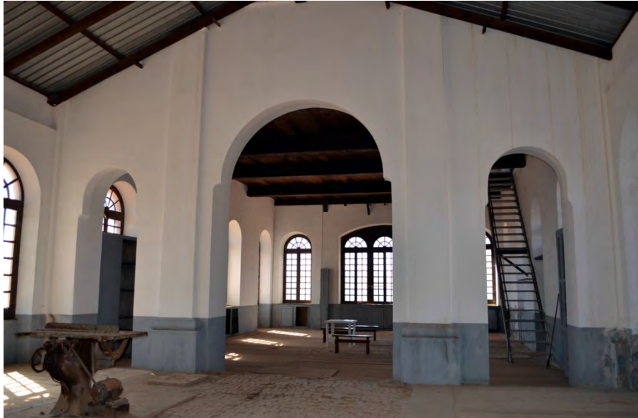
Figure 8. The interior of the carpentry today: the pilasters and arches are those of the original facade. Photo by the author.
