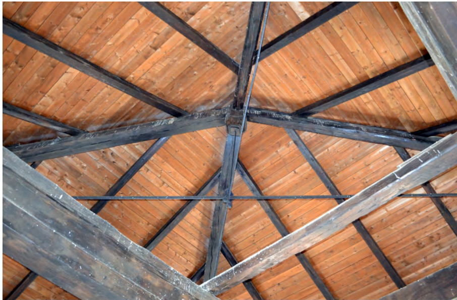
Figure 12. Bottom view of wooden and metal framework of the central volume. Photo by the author.
