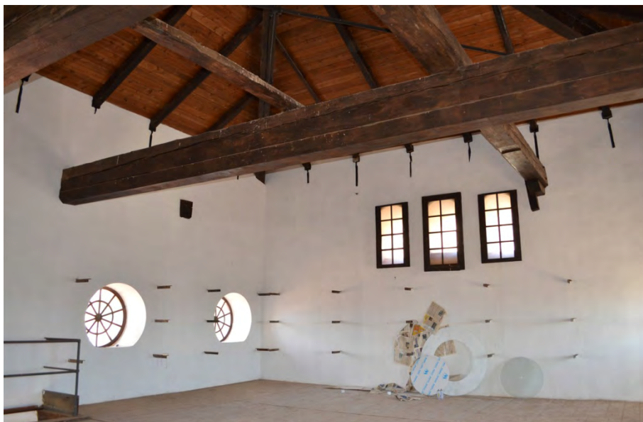
Figure 13. The beams that contain east and west walls of the central body. Photo by the author.
