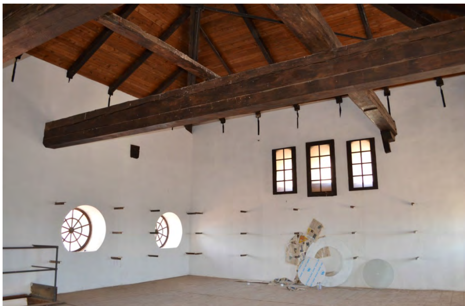
Figure 9. Inside of the central attic with the three recesses in the north. Photo by the author.
