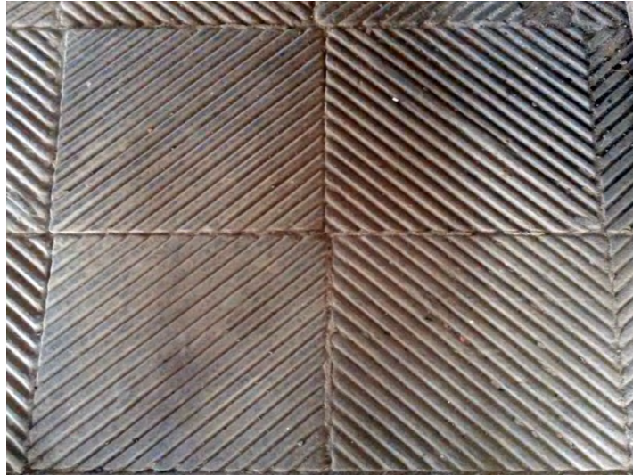
Figure 19. The cast iron plates 50 x 50 in the boiler house. Photo by the author.
