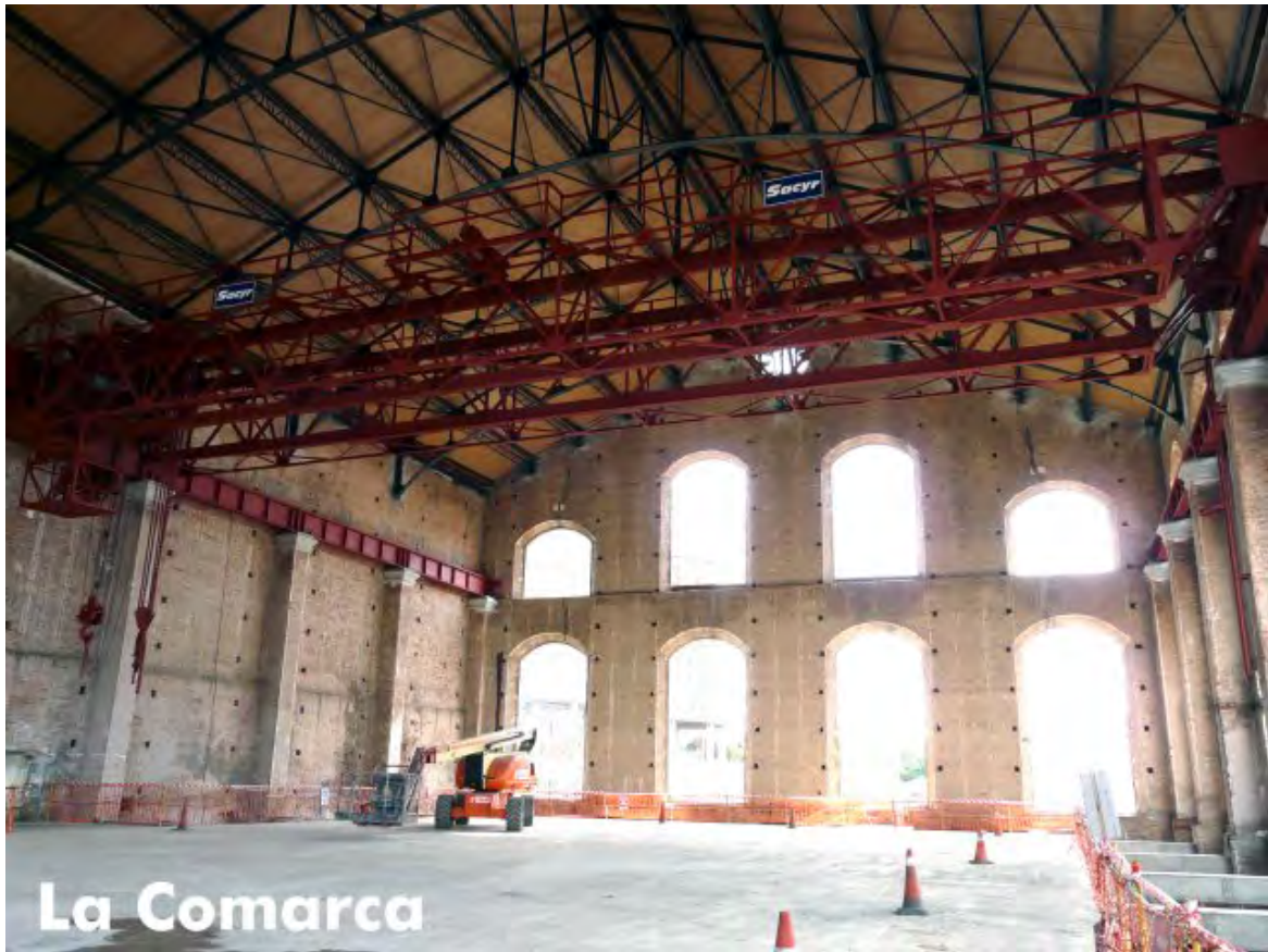
Figure 15. Overview of the interior during works: the metallic bridge present in the roof has been preserved. Source: https://minasdepueblonuevodelterrible.jimdo.com
