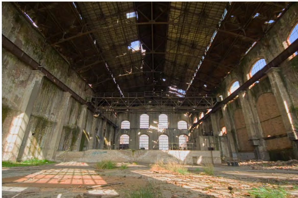
Figure 14. Interior of the Thermoelectric Central in 2008. Source: Javier Callejas on Google Earth.
