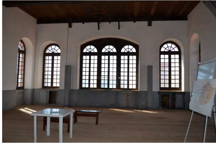
Figure 17. The openings of the carpentry level: the two arched windows and central mullioned window. Photo by the author.
