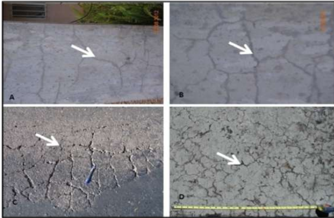
Figure 6-15 Alkali Silica Reaction affected structures (A-D); the effect of Alkali Silica Reaction is well developed in the study area
