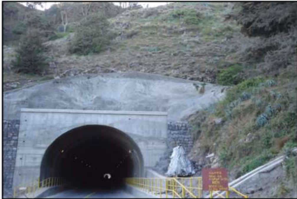
Figure 3-18 Tunnel route (1km long) constructed in the plagioclase porphyritic basalt, the only tunnel way in the country
