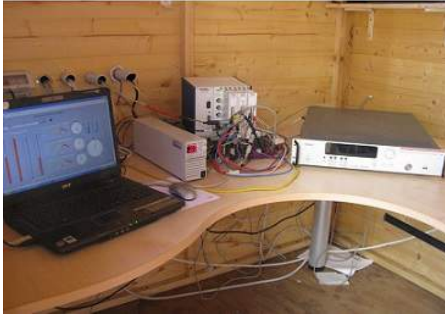
Figure 2.4.3: Acquisition systems in the Sardegna Ricerche outdoor facility.
