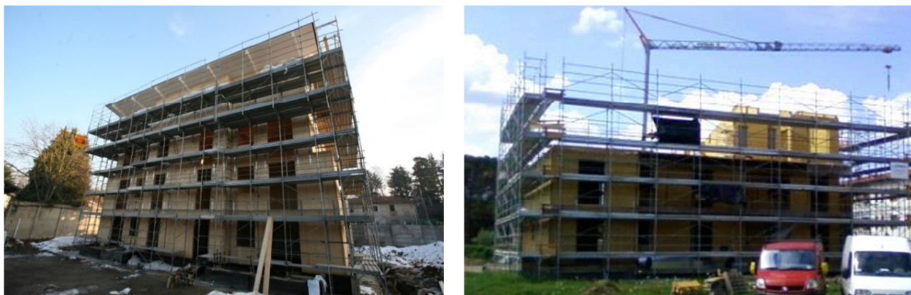
Figure 4-1 Erection of a 4 storey CLT residential building near Varese, Lombardia, northern Italy (left), and of a 3-storey Light-Frame residential building near Lucca, Tuscany, central Italy (right).
