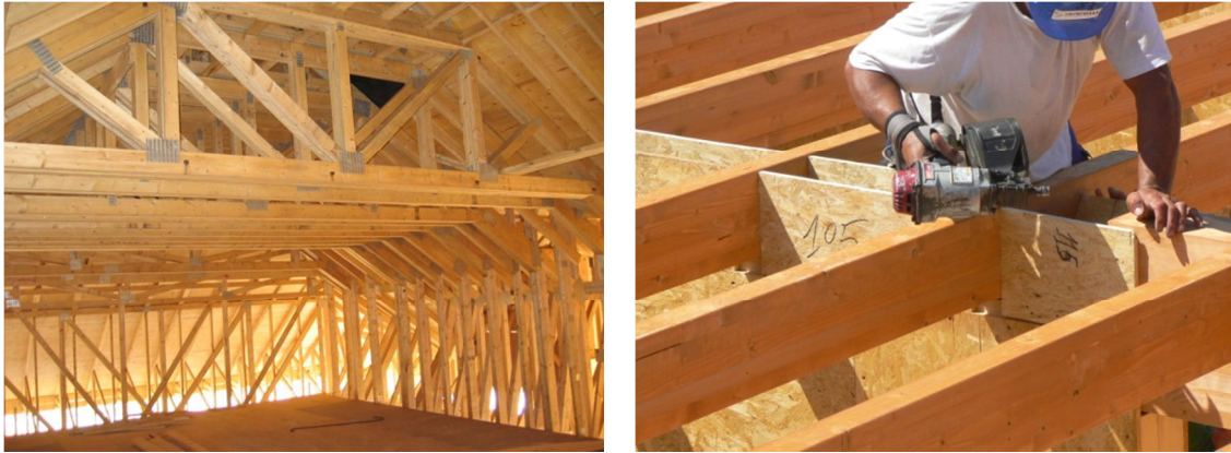
Figure 3-90 Two different types of roof construction: with Light-Frame nailed trusses (left) or with glulam timber beams (right).
