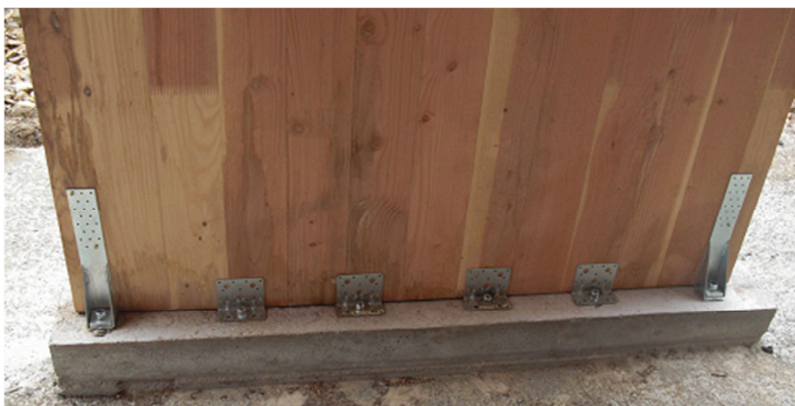
Figure 3-6 Connection of a CLT panel to the foundation with hold-down anchors and steel brackets.
