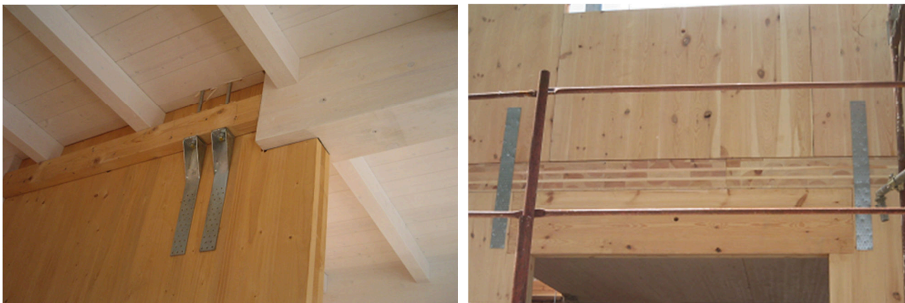
Figure 3-8 Inter-storey hold-down connection for inner walls (Left - in this case two hold-downs below connected to the corresponding two upper hold-downs not visible in this picture) and for external walls (Right) with two nailed steel plates at opening ends.
