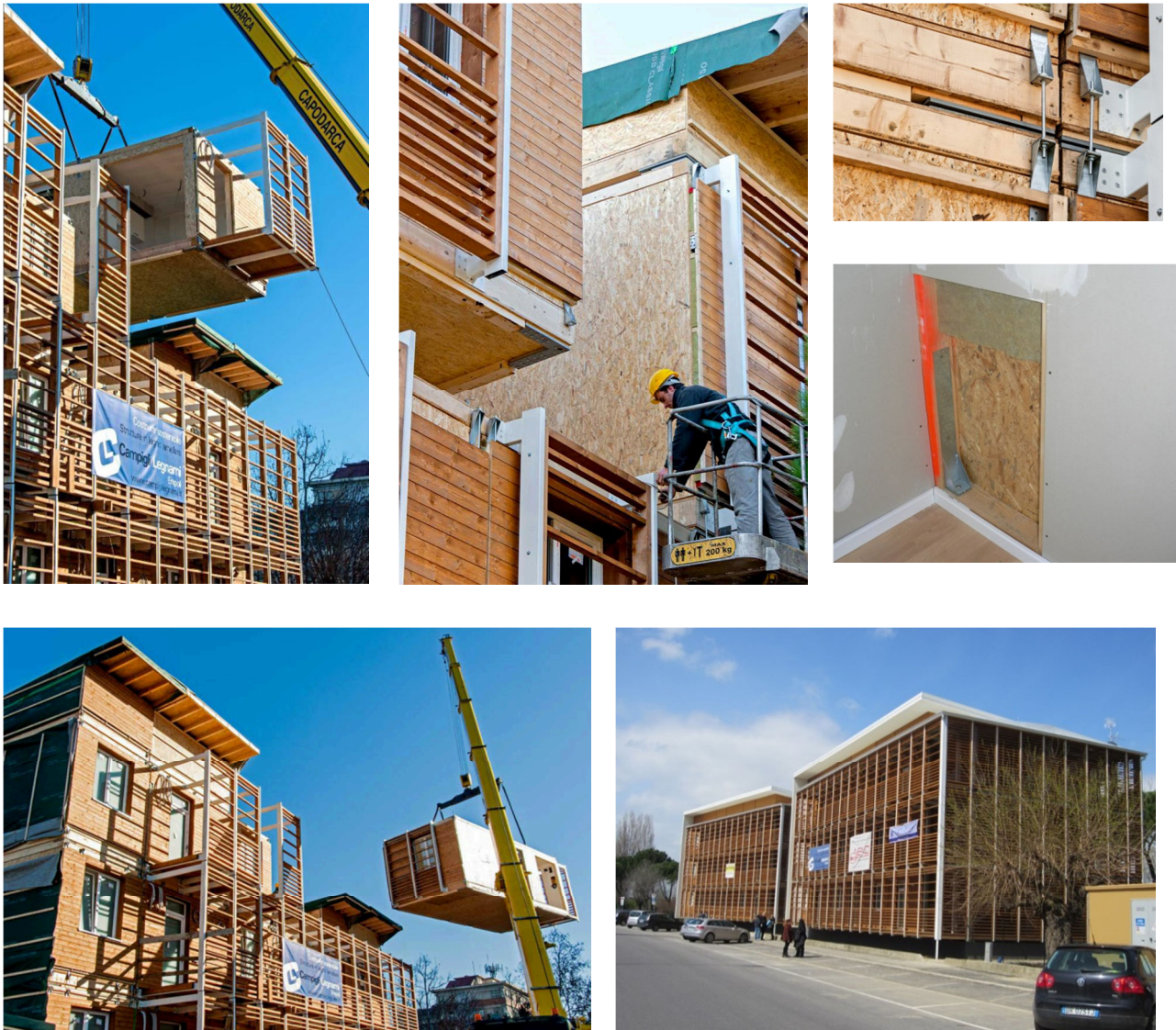
Figure 6-2: Two 3-storey residential demountable buildings built in Florence in 2012. Structural design: dedaLEGNO.
