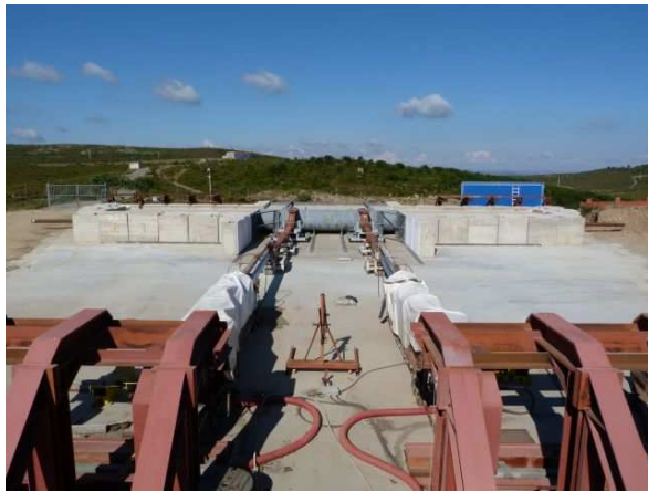
a). Global view of landslide fault equipment.
