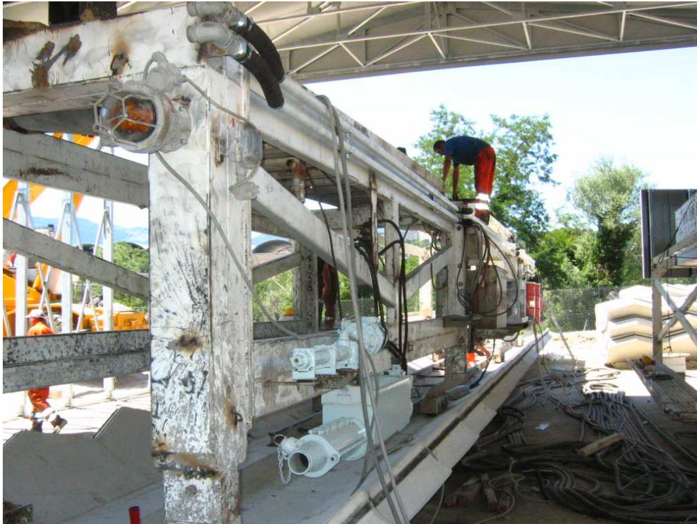
Figura 71: Back up TBM.
