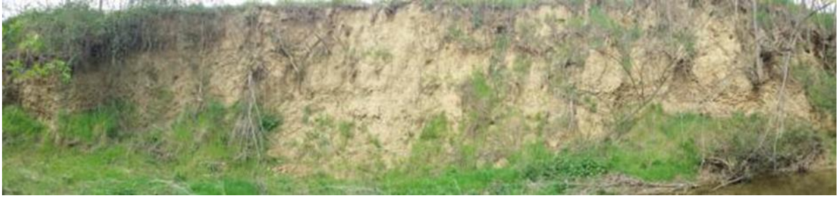
Figure 51 - Panoramic view on the alluvial fan deposit of Bregine River. Are evident lenses of gravel alternated with coarser and fine sand.
