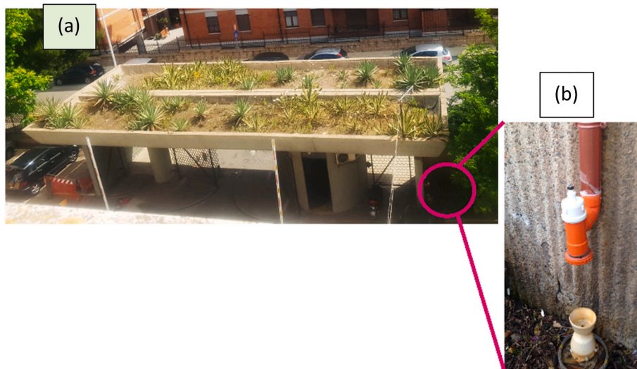
Fig. 2. (a) Top view of the green roof and (b) detail of the water outflow measurement system. (For interpretation of the references to colour in this figure legend, the reader is referred to the Web version of this article.)
