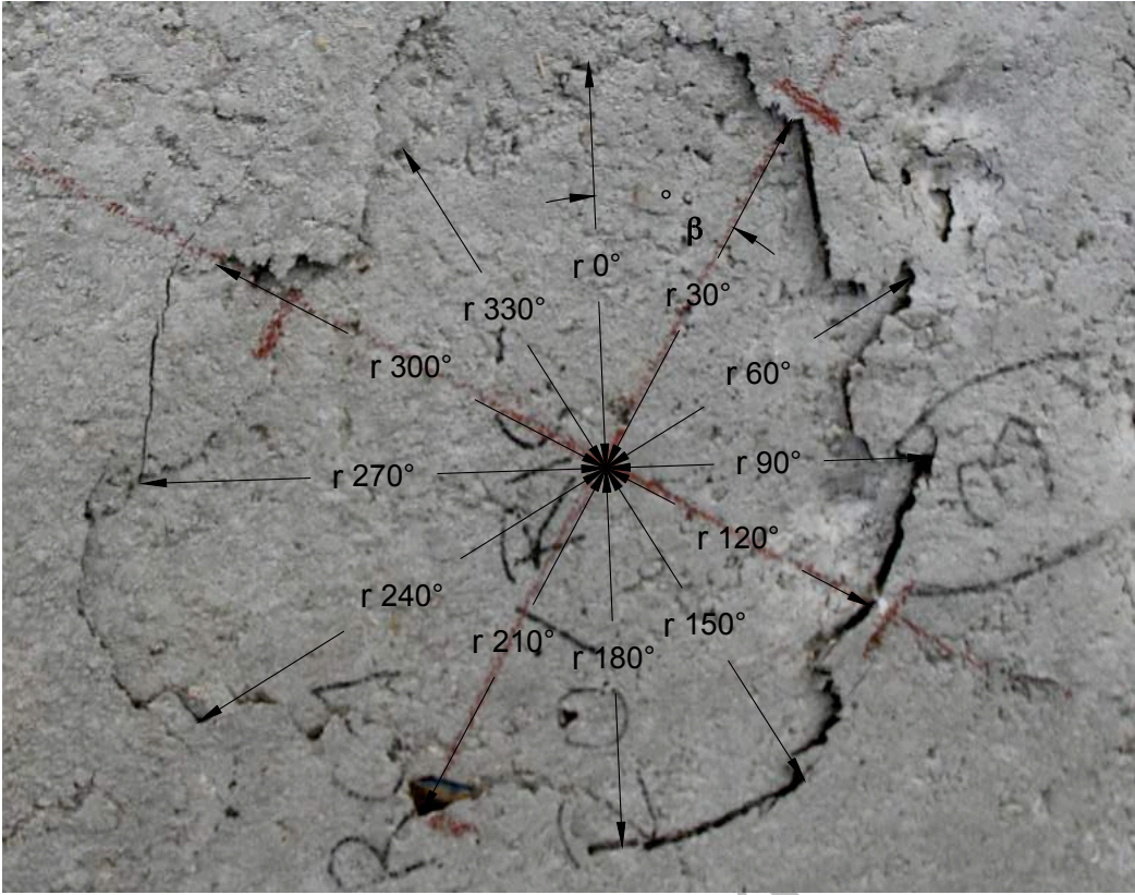
Fig. 8. Top face cracking pattern and radius of the punching cone measured every 30°.
