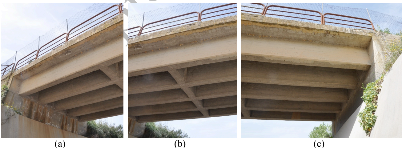
Figure 3. Views of the PC20 bridge conditions, (a) abutment 1, (b) midspan, (c) abutment 2.
