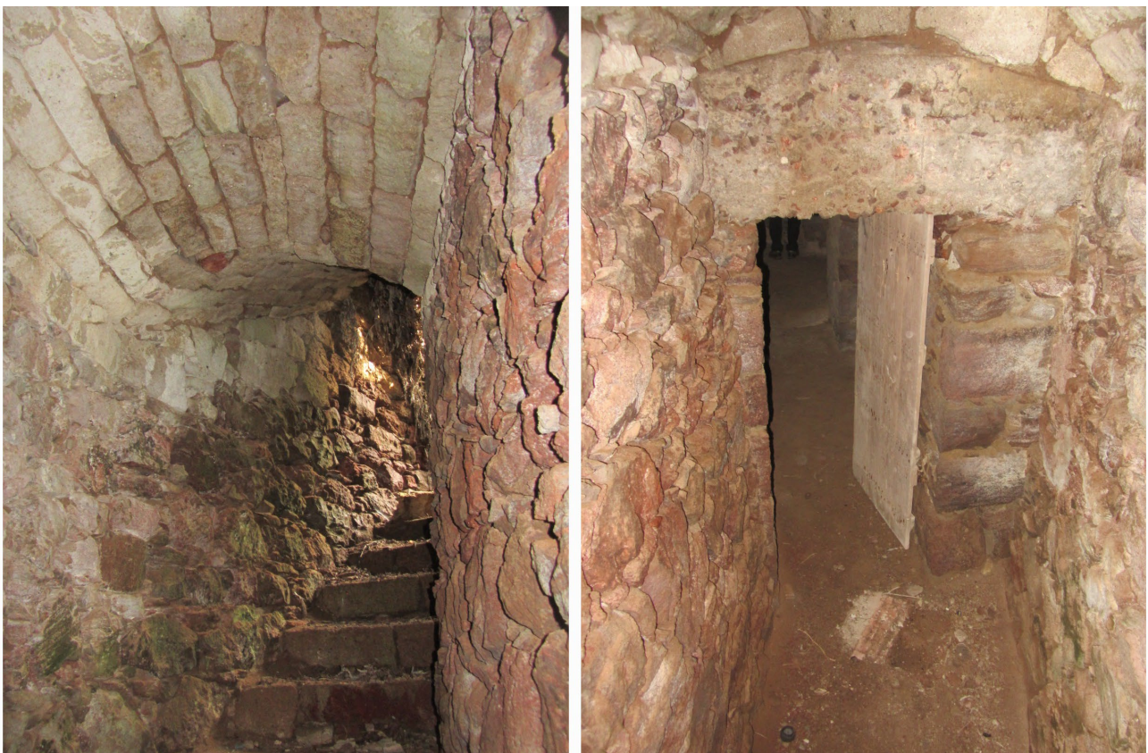
Figure 7. Underground vaulted passage located in the Porto Alabe Beach (Tresnuraghes). The structure, built with local stone, is particularly interesting for the use of traditional techniques integrated with the reinforced concrete.
