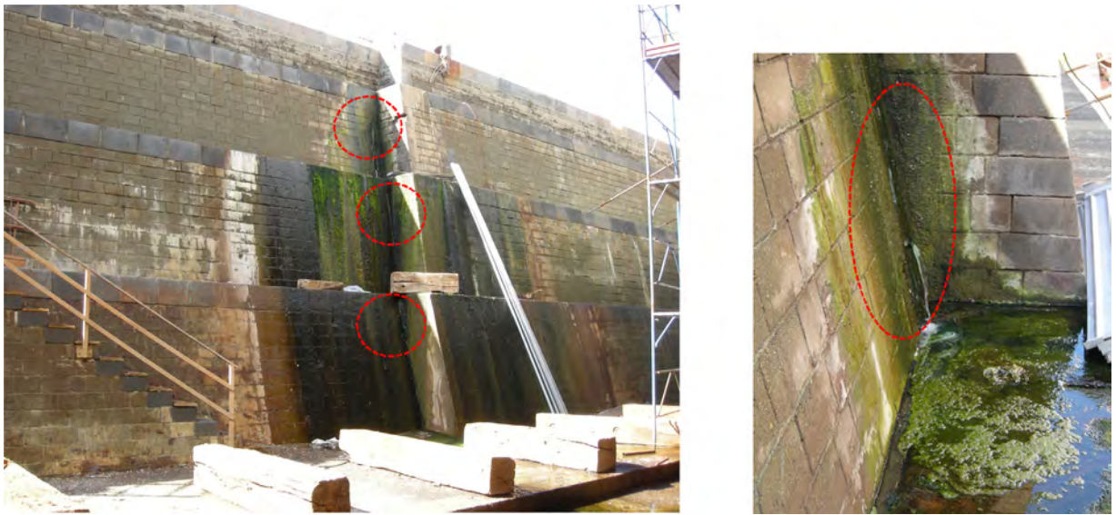
Fig. 26. Existing cracks in walls of Section CC (the most evident in red).
