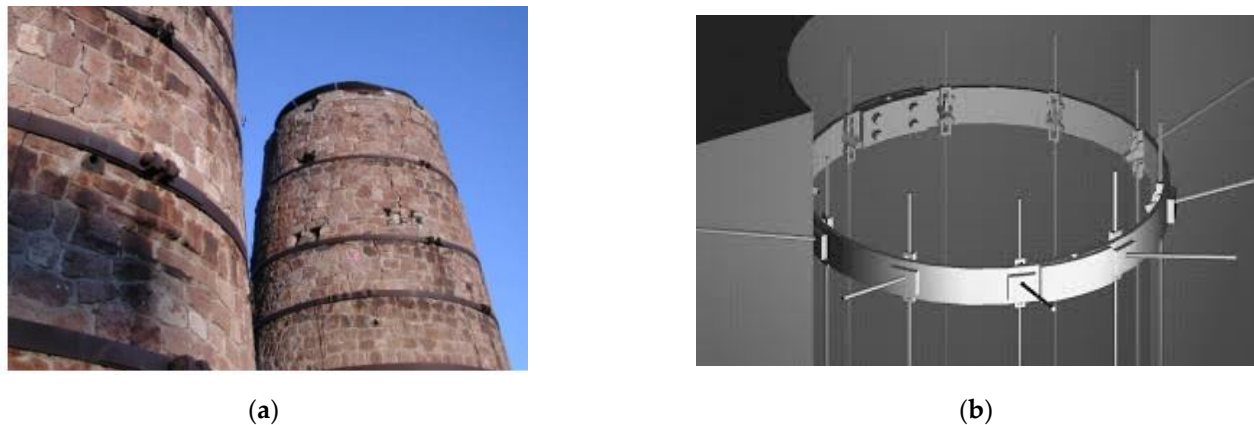
Figure 1. The use of steel reinforcements rings to improve the seismic behavior of slender masonry constructions (invasive modification of the original structure (solution 1)). (a) Outer reinforcement, and (b) inner reinforcement.
