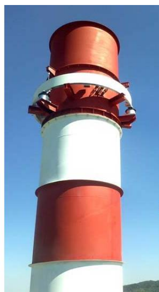
Figure 2. Arquata Scrivia chimney (AL, Italy). An example of applying an auxiliary and reversible system that changes its response under dynamic loads (solution 2).
