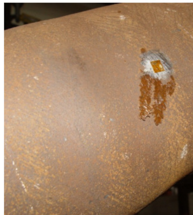
(b) Shear lines on the surface of the compression brace of specimen CFST-6
