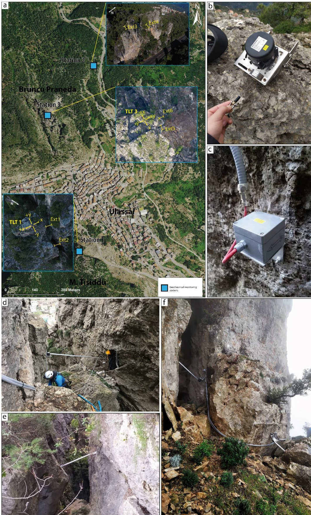
Figure 40 a) Geotechnical station trumentations b) Extensimeter C) Tiltmeter T1; d) Extensimeter Ext 1; e) Extensimeter Ext3; f) Sensor installed in the station 3.
