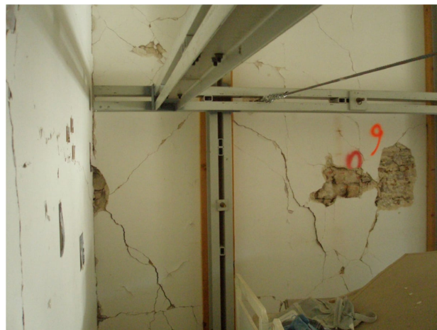
Figure 2. Wall panels with severe cracks.
