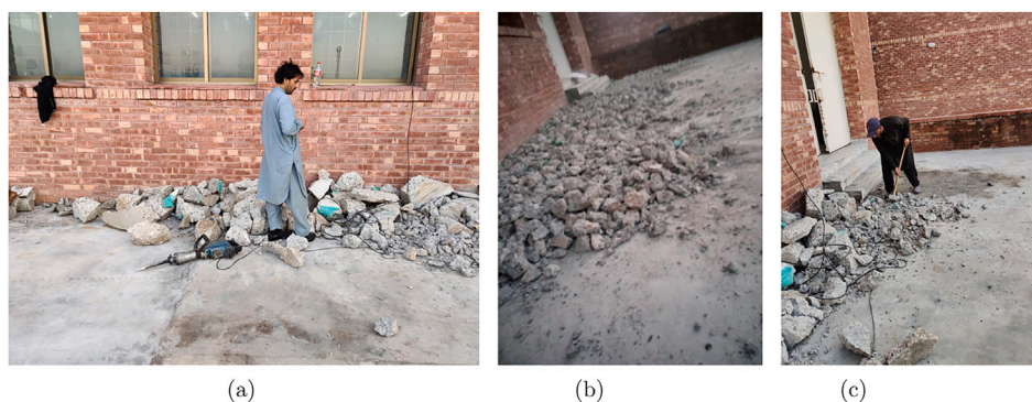
Fig. 2. Processing of demolition concrete waste for the production of recycled coarse aggregates in Pakistan: (a) collection of large concrete debris; (b) crushed material after primary breaking; (c) manual sorting before sieve processing.
