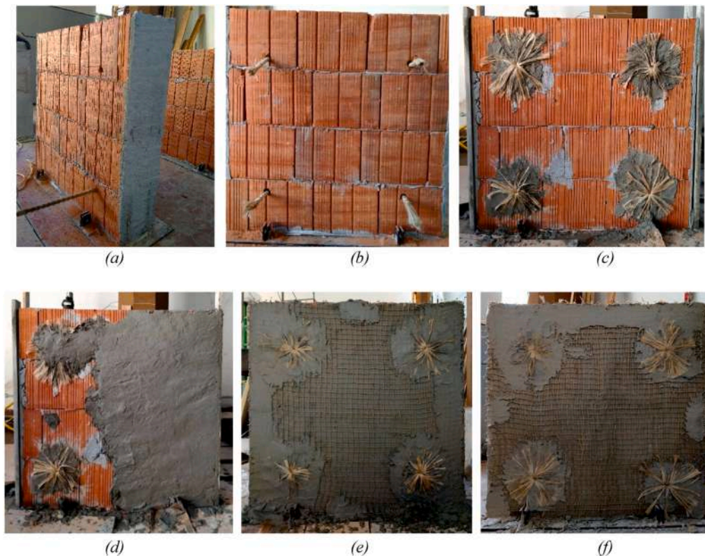
Fig. 14. Retrofitted/upgraded masonry walls: (a) Drilling transversal holes, (b) diatons placed through the masonry wall, (b) diatons are installed and fixed on the masonry wall, (c) application of composite mortar on the masonry wall, (d) jute net (2.5 cm × 2.5 cm mesh configuration) and jute diaton application on masonry wall, and (e) jute net (1.25 cm × 2.5 cm mesh configuration) and jute diaton application on masonry wall.
